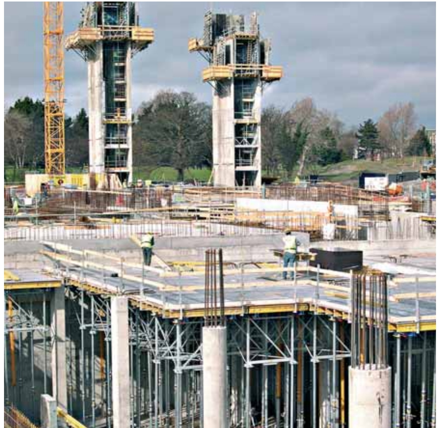
The stair cores are being formed ahead of the main building frames, using Framax framed formwork and the MF 240 system. Dokaflex and Dokamatic tables are in use for the floor-slabs. Undertable support heights of up to 6.80 m are achieved by adding Dokamatic table frames.
