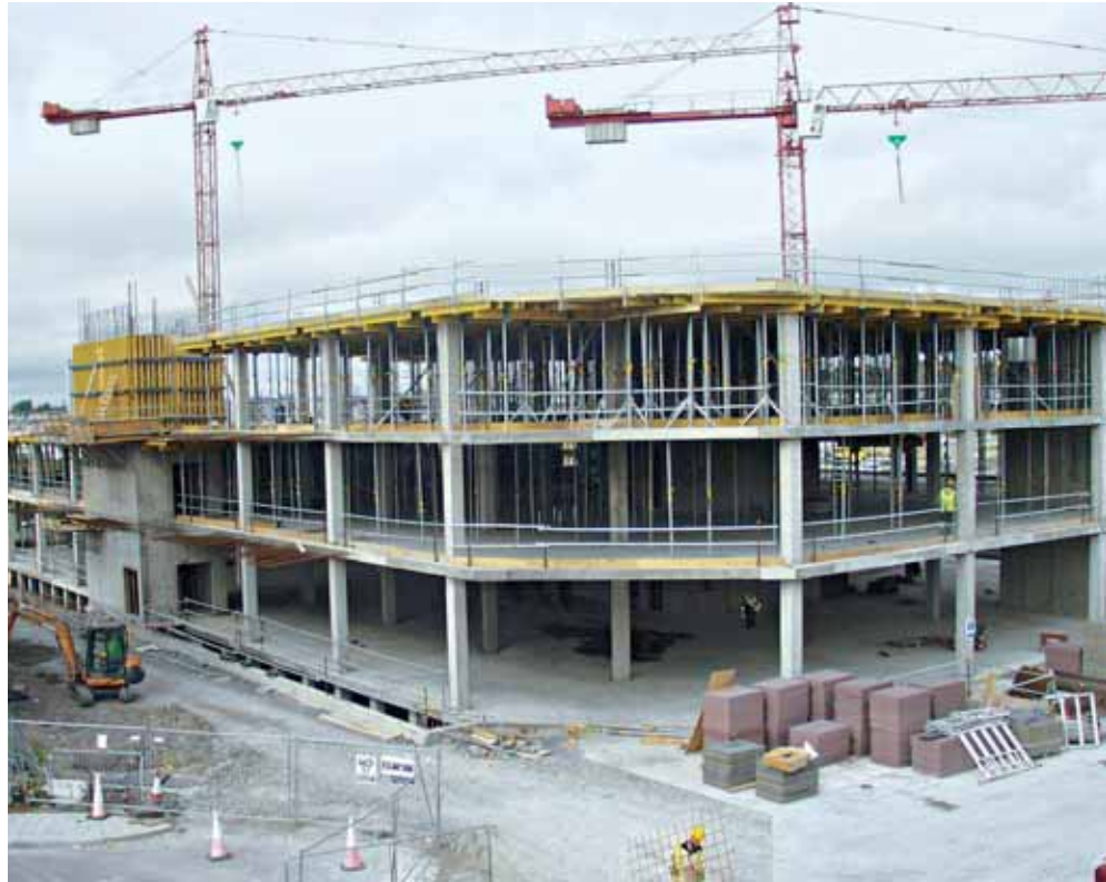
Shannon Formwork successfully used Dokaflex Tables during the construction of the Dell Computer HQ in Cherrywood, County Dublin.
