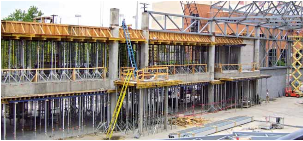
Over 18,000 sq. ft. of Dokamatic Tables were used to complete the 1st level in two pours.
