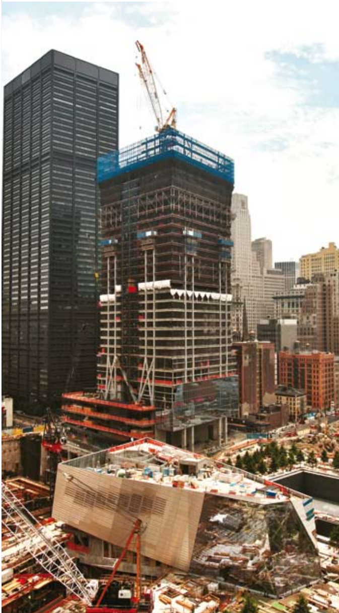
▲ Tower 4 is a structural steel-framed building. Framing the steel takes place approximately six-to-eight stories above the pouring of the concrete core and mega-columns. The steel erectors must provide shielding to protect workers below, as crane picks are not allowed directly into the building. To work within these constraints, Doka is hydraulically climbing everything within the core.
