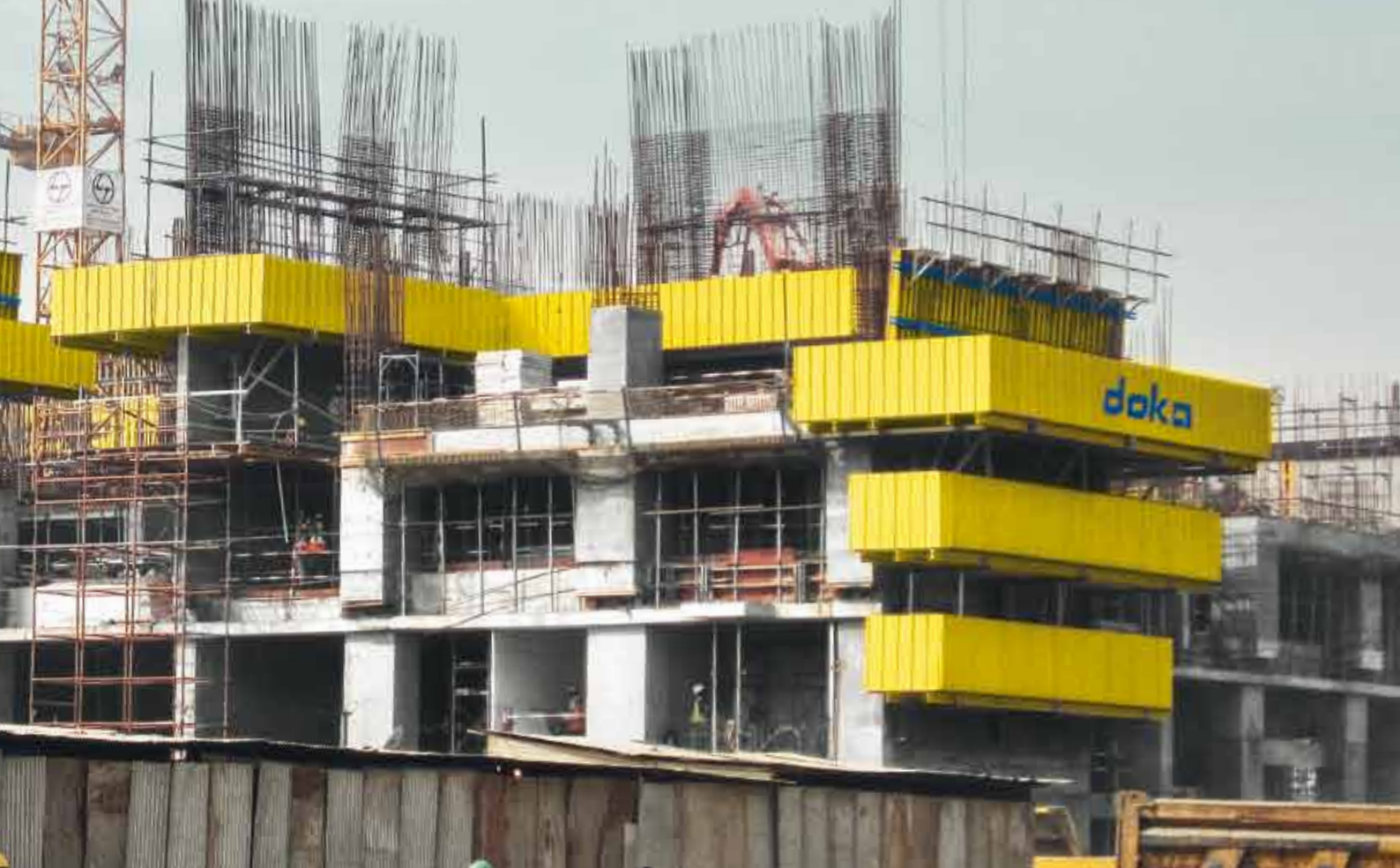
▲ Wadala Towers, soon to stand as a national recognition! Working platforms are one of the most important safety measures taken by Doka for those working at greater height.
