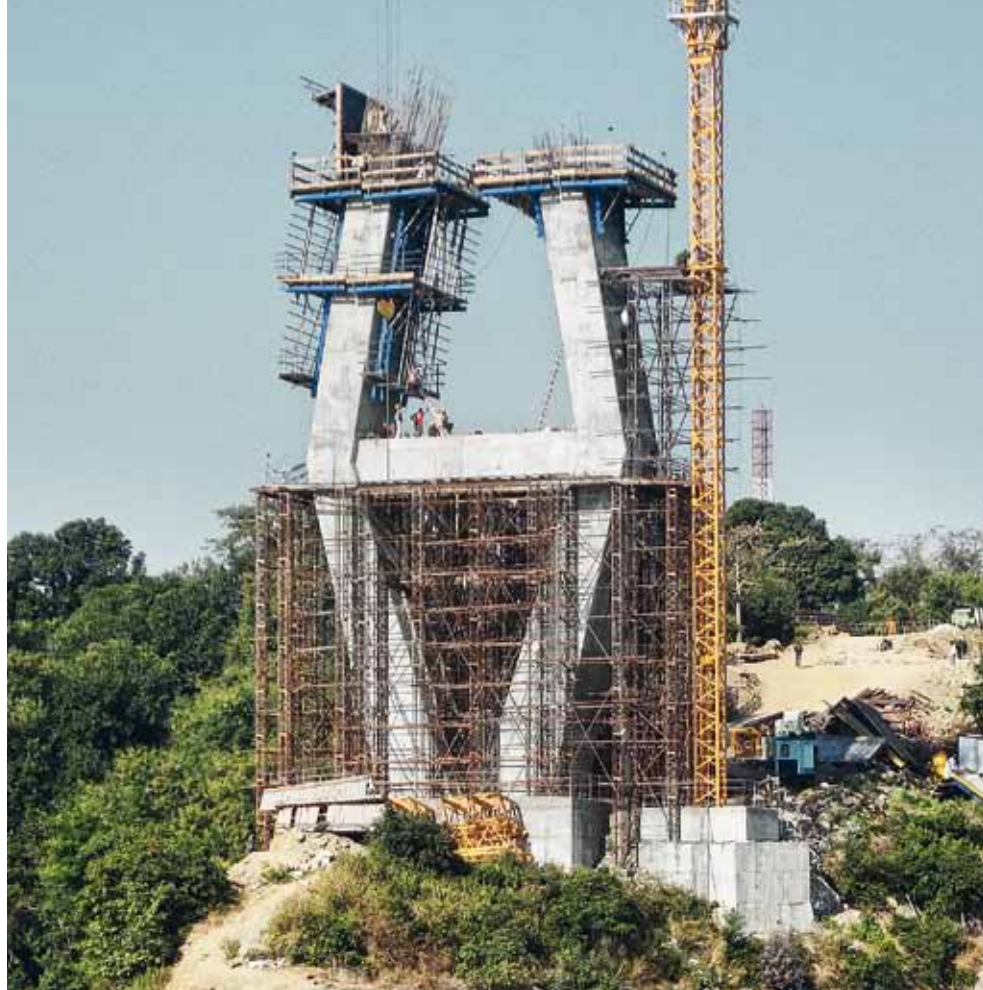
▲ Novel stability, in effect – Doka's solutions are not only designed from the operational point of view, it also ensures the safety of the site crew in face of erratic weather conditions.
