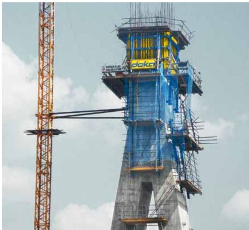
▲ Nuances of a sturdy foundation – Doka India has supplied formwork solutions like Climbing formwork MF240 for the base of the pylon, and Automatic Climbing formwork Xclimb 60 for the upper part of the diamond shape, which will also be used for the straight part of the pylon. Both the formwork variants are adaptable to the structure lending flexibility and versatility to the entire system.
