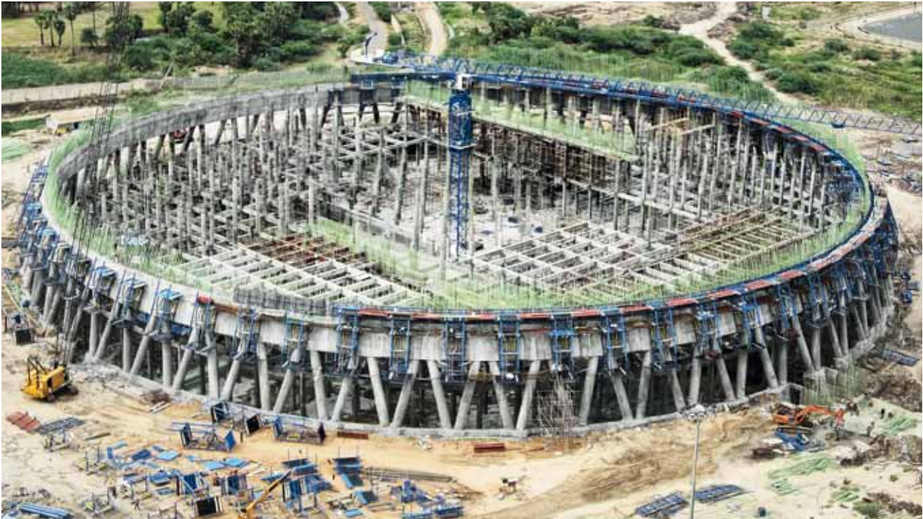
▲ The cooling-tower formwork adapts easily and quickly to the tower's changing cross-section, and the adjustments are carried out from the platforms.
