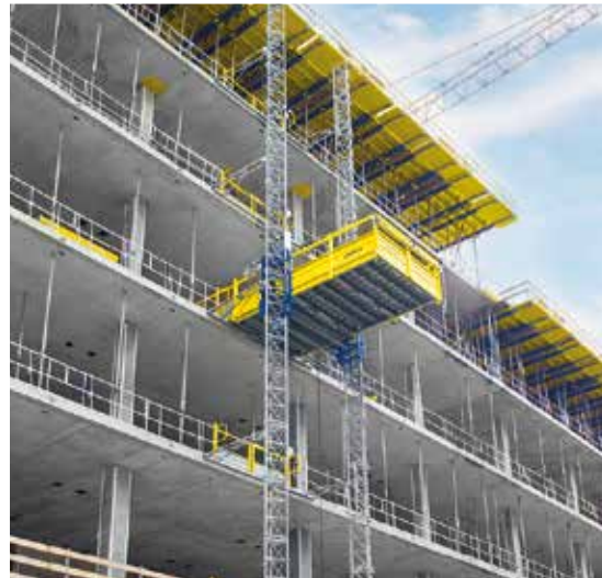
Fast construction workflows without the crane: with the Table Lifting System TLS, tableforms are brought up to the next floor at the push of a button.
