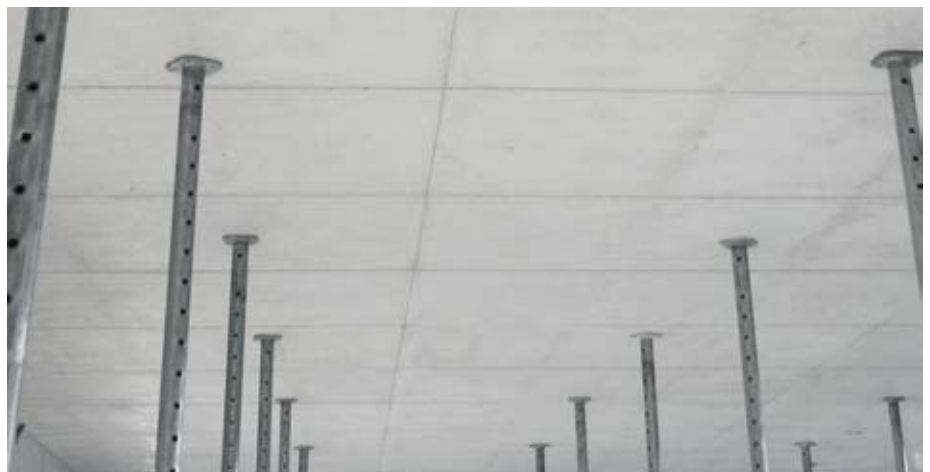
Slab undersides looking good: The Xlife sheeting makes for smooth surfaces; the framing produces a clean, aesthetically appealing join pattern.
