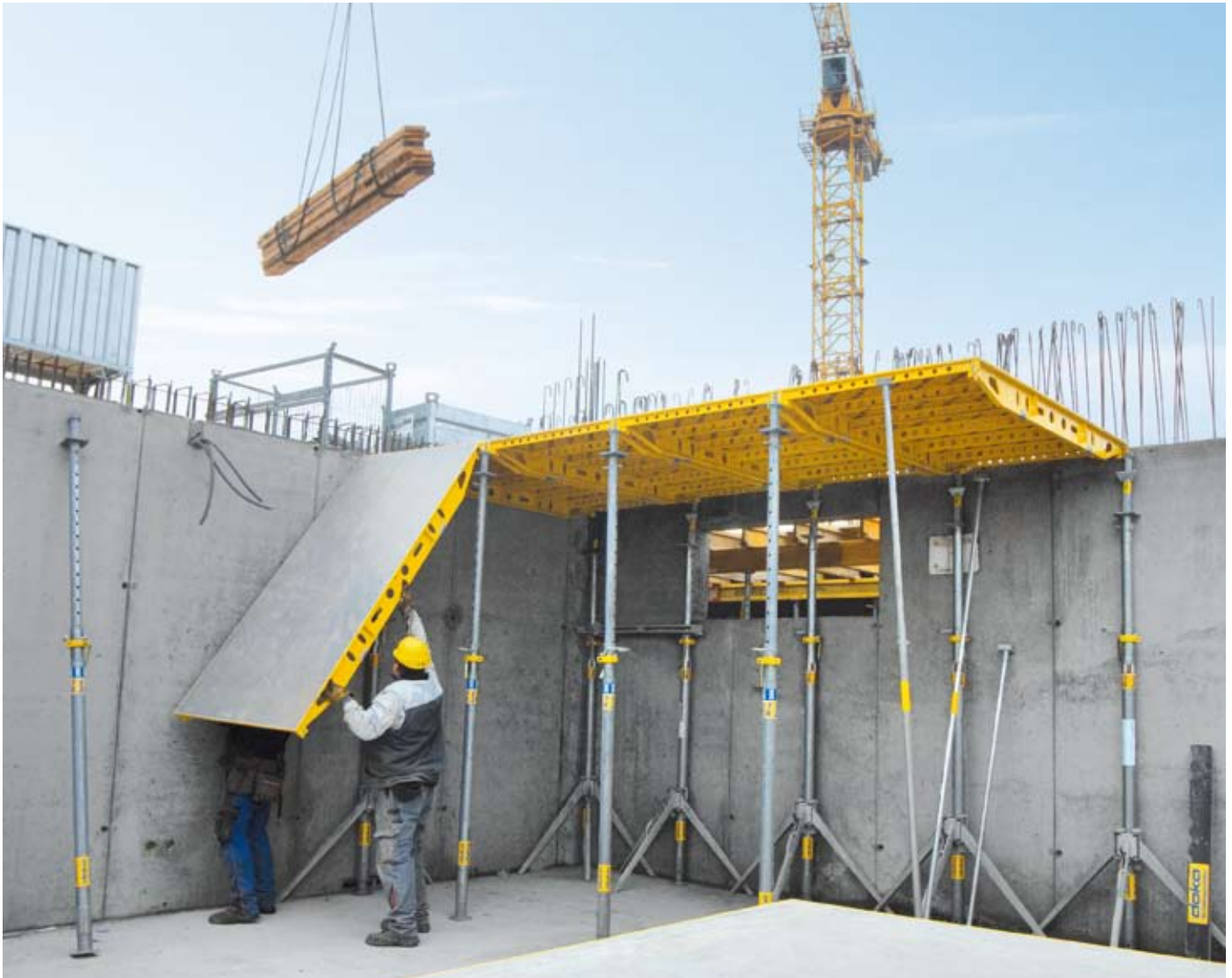
Handsetting from the safety of floor level: Valuable crane capacity is freed, so craneage is available for other tasks to speed up site progress.
