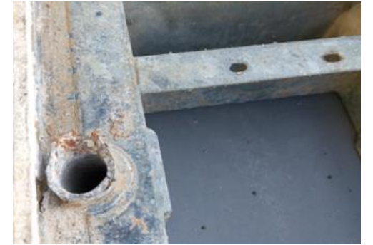
Missing or damaged anchor protection
