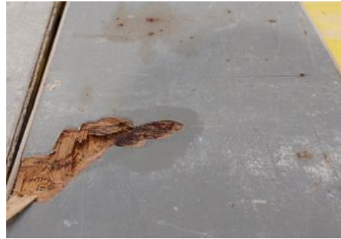
Plywood crack > 10 cm length
