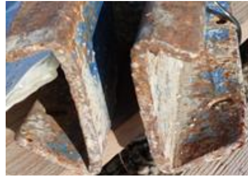
Twisted and deformed > 5mm
