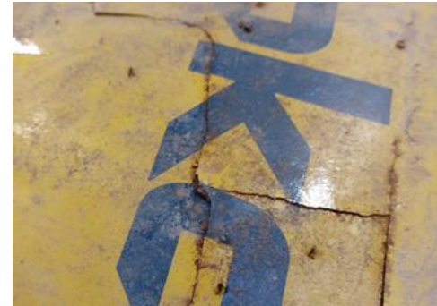
Plywood crack > 10 cm length
