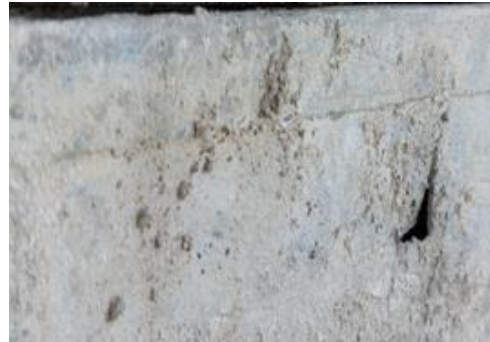
Hole in profile – weld needed
