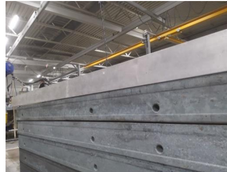
Panel bent / panel deformation
