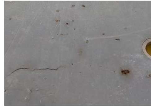
Plywood crack > 10 cm length
