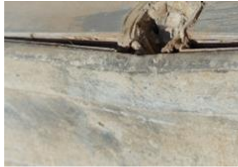
Anchor hole damaged and length profile twisted
