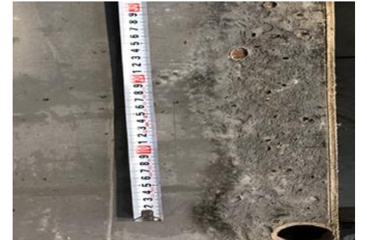
Burned plywood = 10 cm
