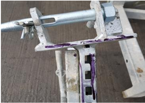
Connecting part to bracket broken/bent
