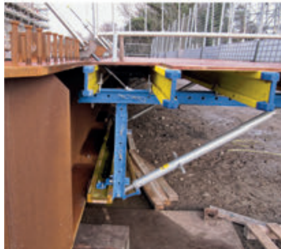
This versatile cantilever arm formwork is attached to the bridge superstructure by means of re-useable diagonal anchors.
