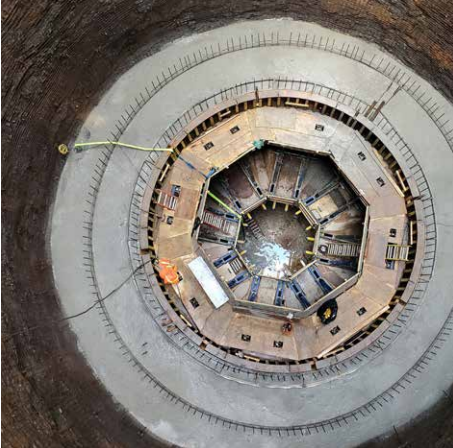
With the use of DokaXact for a sanitary sewer shaft in Mississauga, Ontario, pouring time was reduced by 5 hours.
