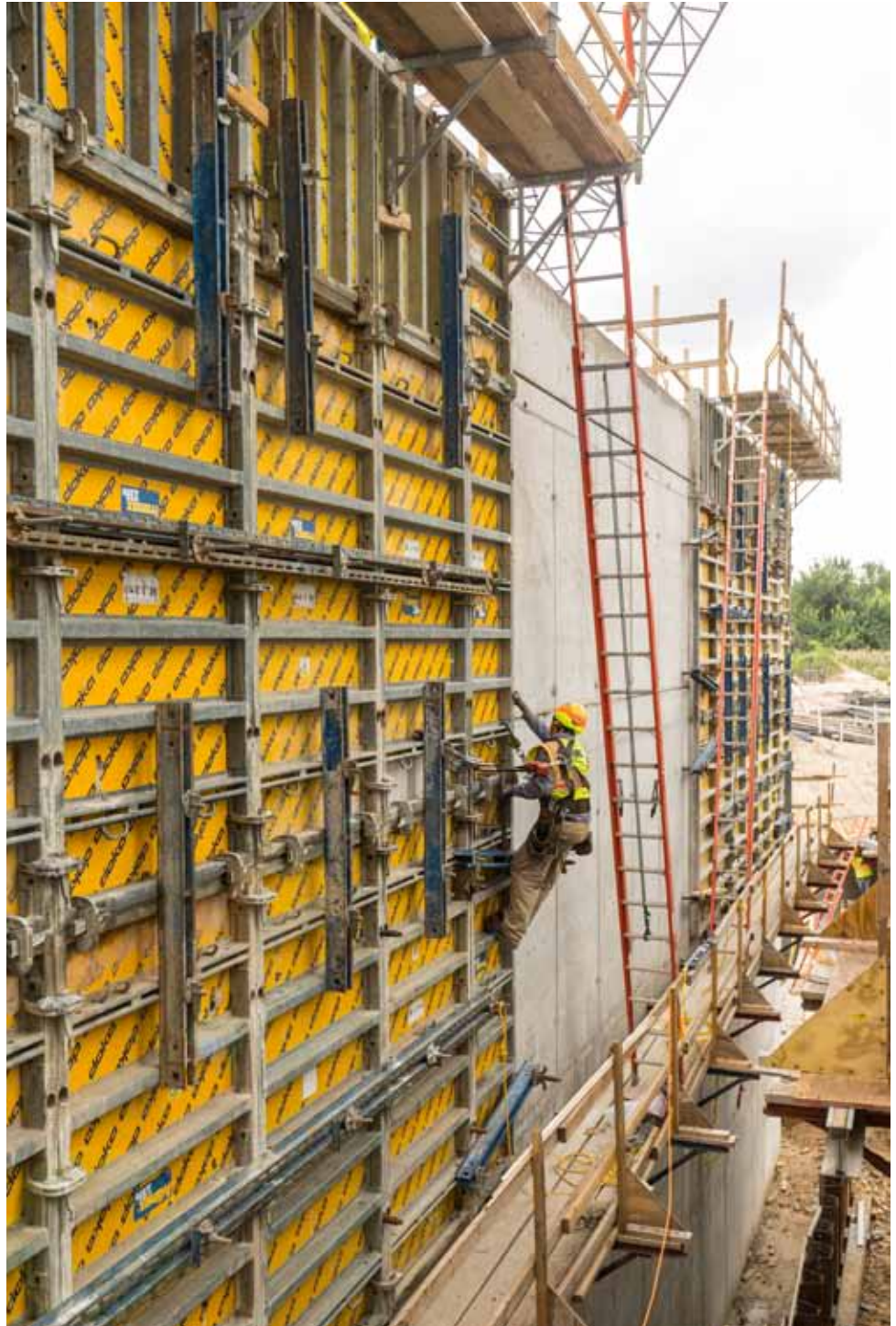
▲ The contractor used both Framax and Frami Xlife formwork for the five-foot-thick base mats, and Frami with steel channels for the troughs.
