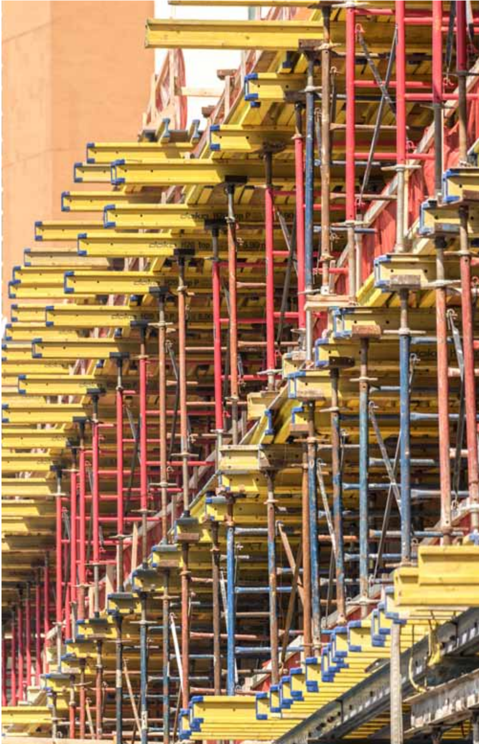
▲ Doka’s 10 kip shoring was used on the 2nd and 5th floor levels.
