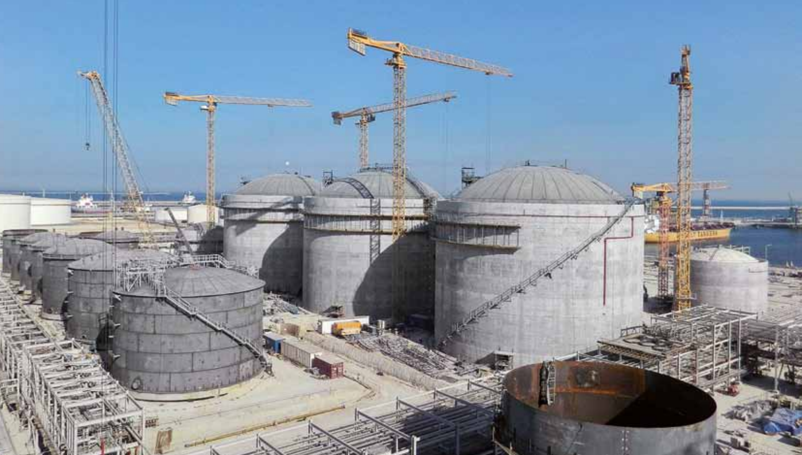
▲ Doka is forming 44 tanks as part of what will be the world's largest petrochemical industrial complex.
