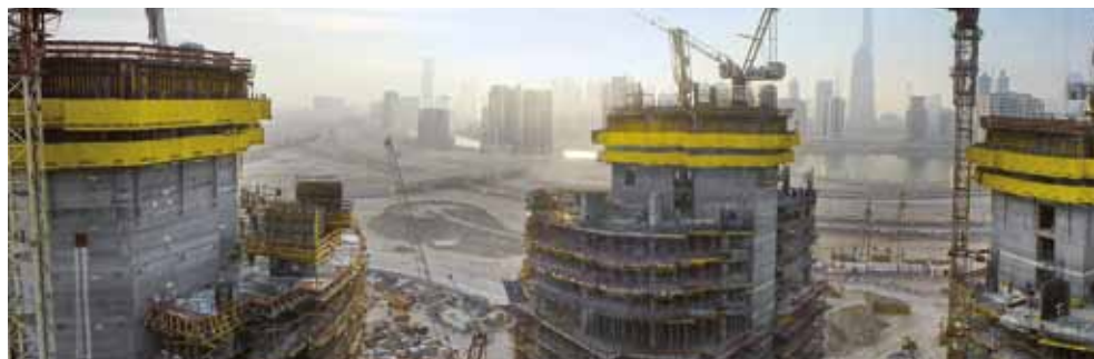
▲ Doka convinced the customer with a tailored formwork solution for the tight schedule and limited storage space on site.
