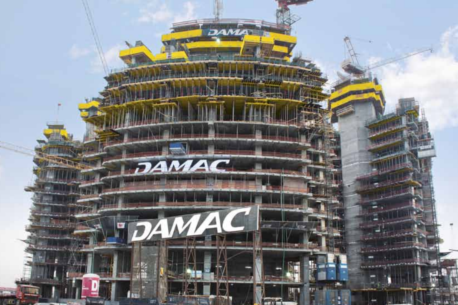
▲ The Paramount Hotels and Resorts project comprises one hotel and three residential towers.
