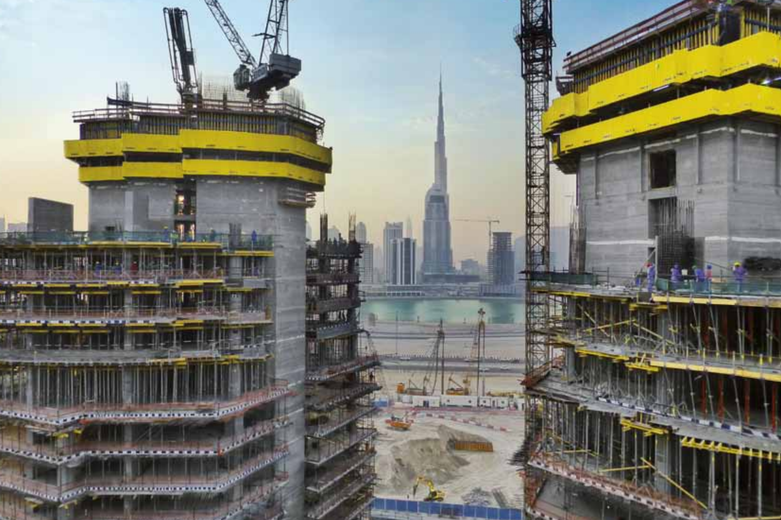
▲ The crane independent Automatic climbing formwork SKE50 ensures a successful corewall assembly.
