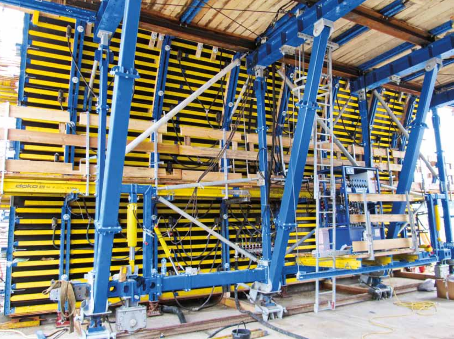
▲ DokaCC is an innovation especially for the cut & cover construction method used in tunnels: quick, efficient and safe.
