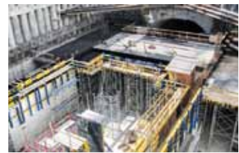
▲ Even architectural demands such as with the Metro expansion in Algeria are realised quickly and safely with high-performing Doka products.
