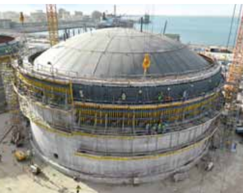
▲ Using the high-performing Doka climbing formwork 150F facilitates pouring a 3.45-m section per week.
