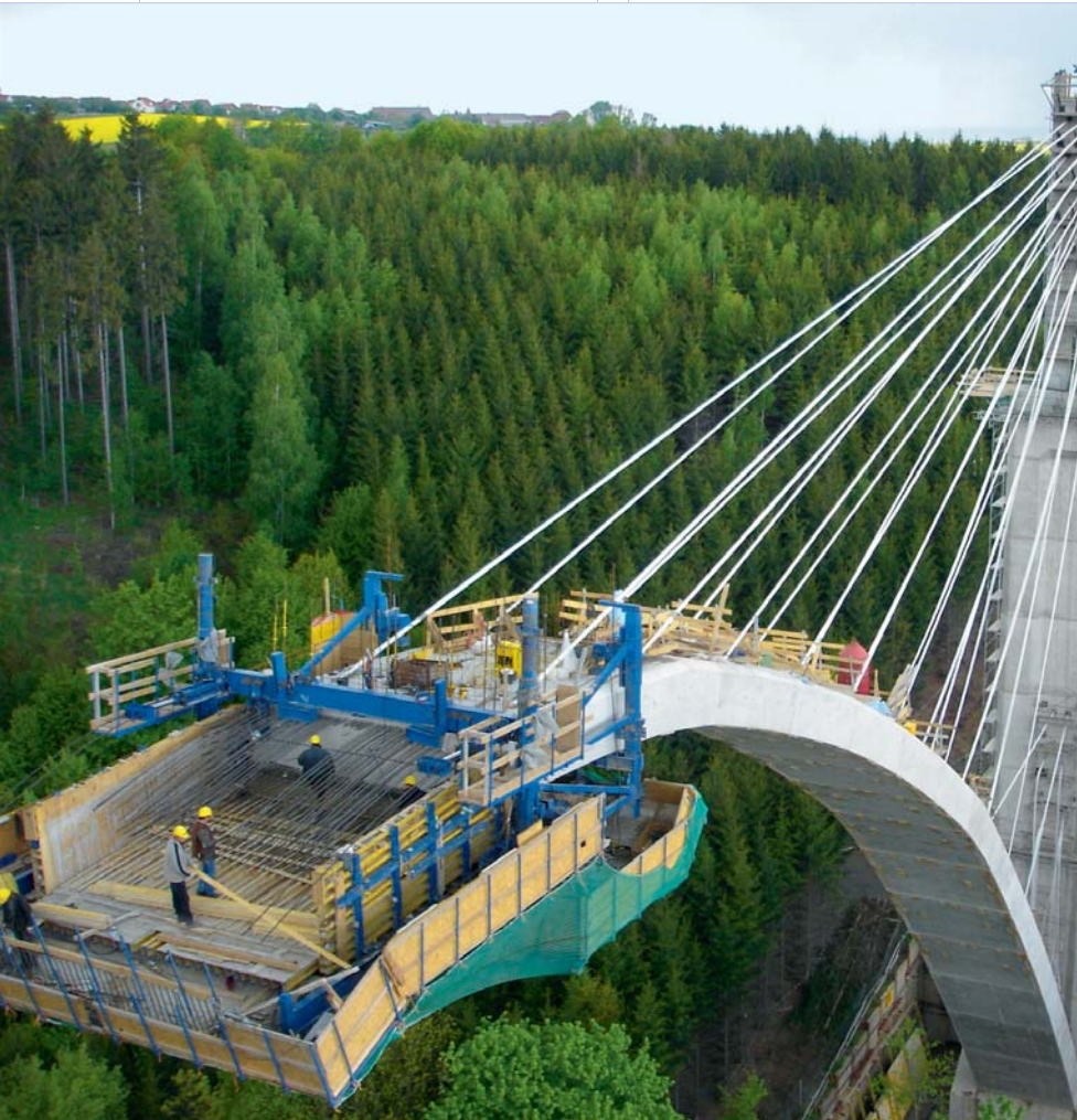
◀ The Seidewitztal Bridge in Germany was built with the Doka forming traveller.
