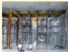
Taoyuan Airport, Taiwan
