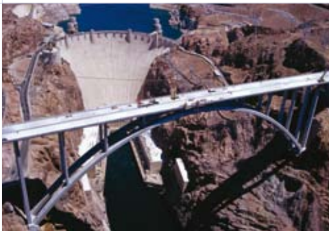
▲ The construction of the Hoover Dam Bypass Bridge involved a series of inventive solutions to provide efficiency on the jobsite. Doka supplied Framax Framed Formwork to pour large anchor footings for the massive cranes. This equipment then was moved over the canyon's edge and reused to pour the pier footings and abutments. The innovative design layout saved the contractor the cost of multiple sets of forms.
