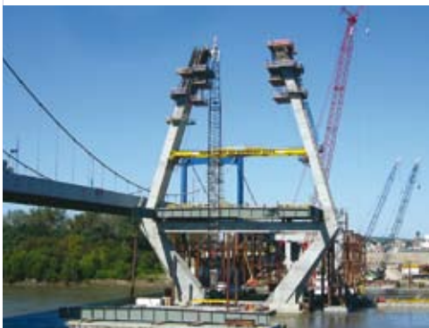
▲ Doka was selected to provide the engineering solutions and formwork for the top half of the bridge pylon on the 260-ft. high Paseo Bridge in Kansas City. Because of the
