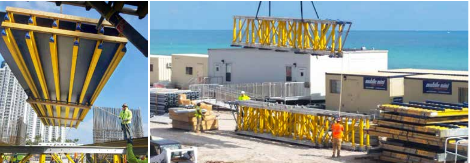
Preassembly of Doka Truss Tables onsite shows leg braces and table tops with plywood beign flown on them.
