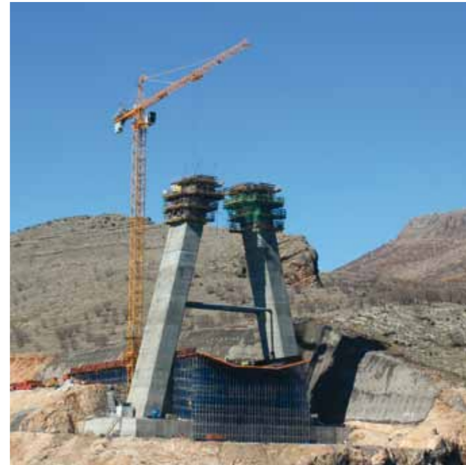
The Nissibi Bridge is being constructed across the Euphrates in South Anatolia. The cable-stayed bridge is 610 metres long and is supported by 85-metre-high pylons.
