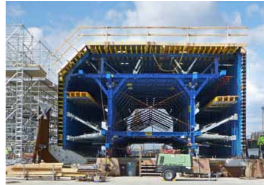
"Engineered by Doka" is a seal of quality for international showcase projects like the Second Midtown Tunnel, an immersed tunnel in the United States.
