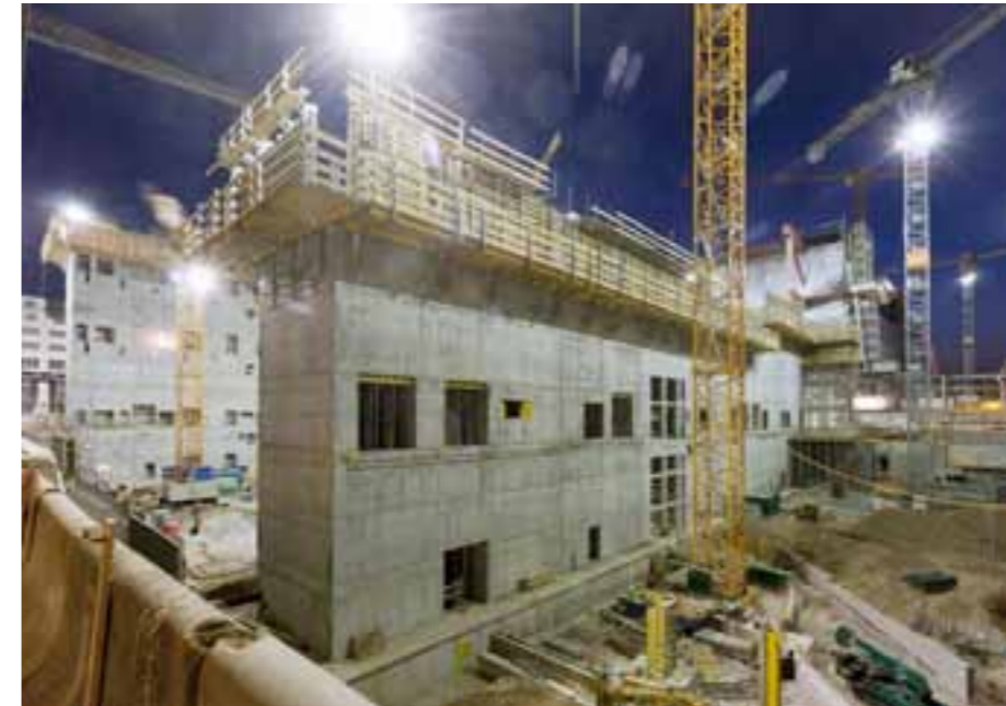
The trade fair grounds in Basel are undergoing a notable modernisation. Doka Switzerland is supplying, among other things, the formwork technology for a new building with three floors of exhibition space and an event hall.
