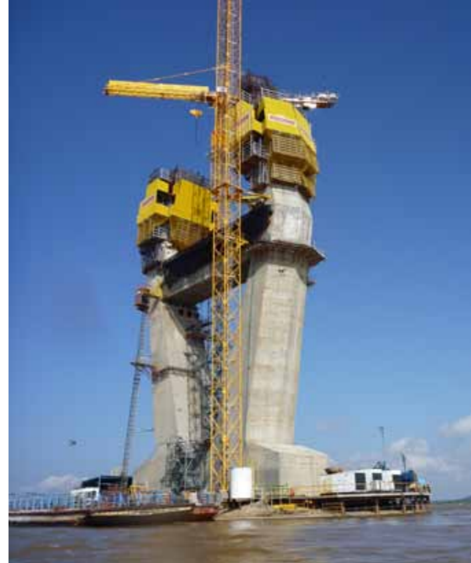
On the banks of the Orinoco in Venezuela, two pylons are being constructed with the help of a formwork solution by Doka.
