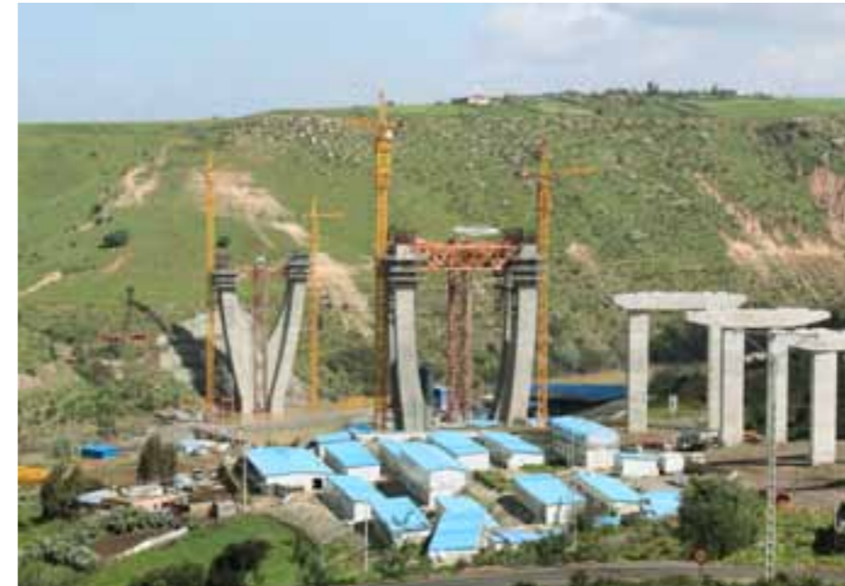
The Bouregreg Bridge is an example of international cooperation and complexity. With this showcase project Morocco hopes to make the transition to the infrastructure of tomorrow.
