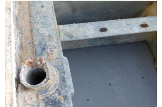
Missing or damaged anchor protection
