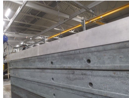
Panel bent / panel deformation
