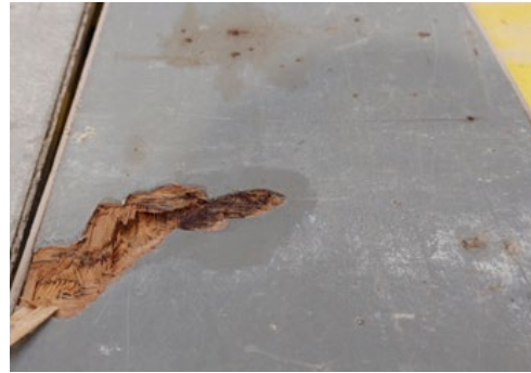
Plywood crack > 10 cm length
