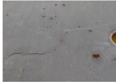
Plywood crack > 10 cm length
