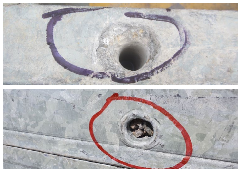
Profile anchor holes damaged or filled with concrete
