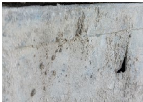
Hole in profile – weld needed
