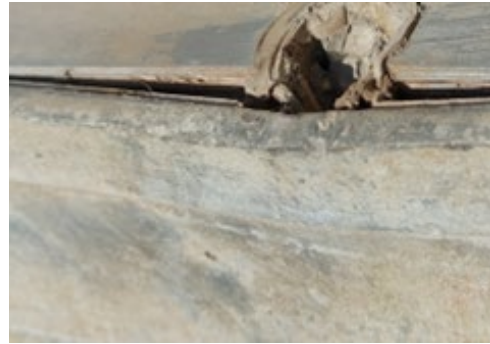
Anchor hole damaged and length profile twisted
