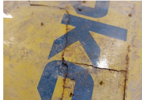
Plywood crack > 10 cm length
