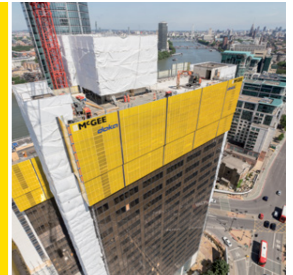
No. 1 Nine Elms , London, UK | 89 m: Automatic downward climbing with noise-abatement enclosure for controlled demolition work
